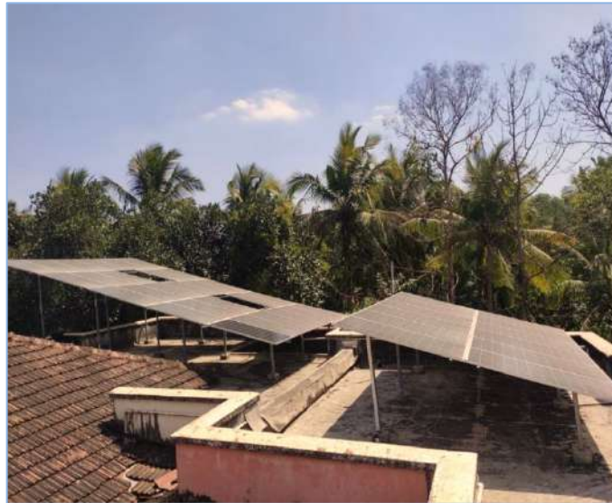
PV solar panel installed at Quepem Health centre, Goa
