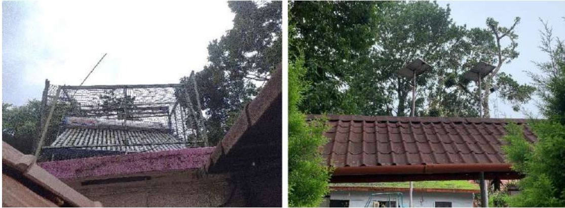
Solar powered water heating and outdoor lighting facility at Noolpuzha FHC, Kerala
