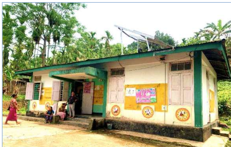
Solar panels installed at Darugre sub-centre
