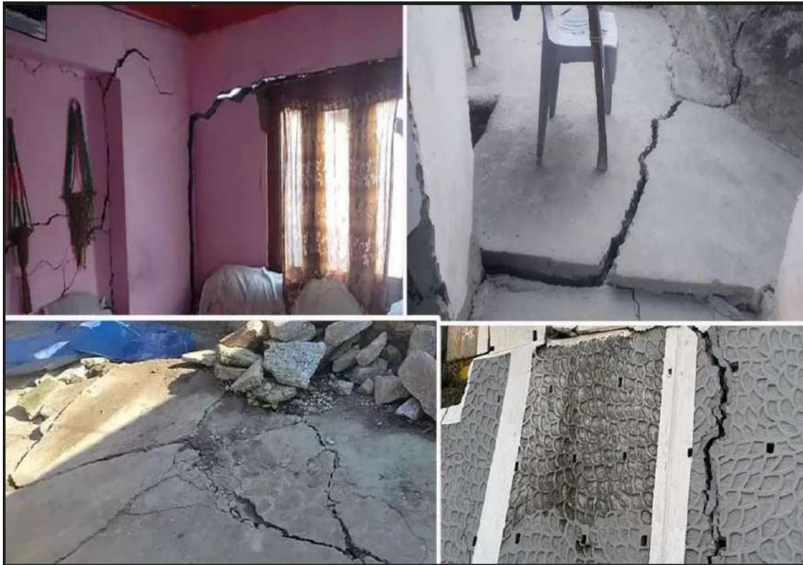
Pictures of Land subsidence - Joshimath, District Chamoli, Uttarakhand, India
