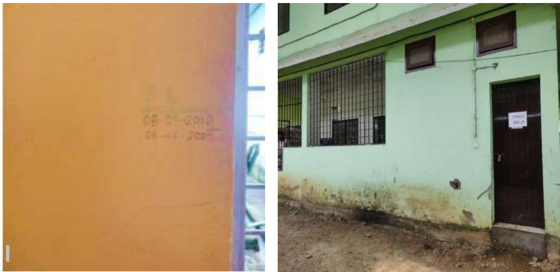
(Left) Flood water levels marked on the wall, (Right) Dirt in walls due to flooding, Vandiperiyar CHC
