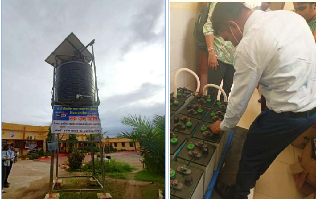
(Left) Water tank connected to Solar Panels (Right) batteries of solar placed in a separate room, Patewa PHC, Chhattisgarh
